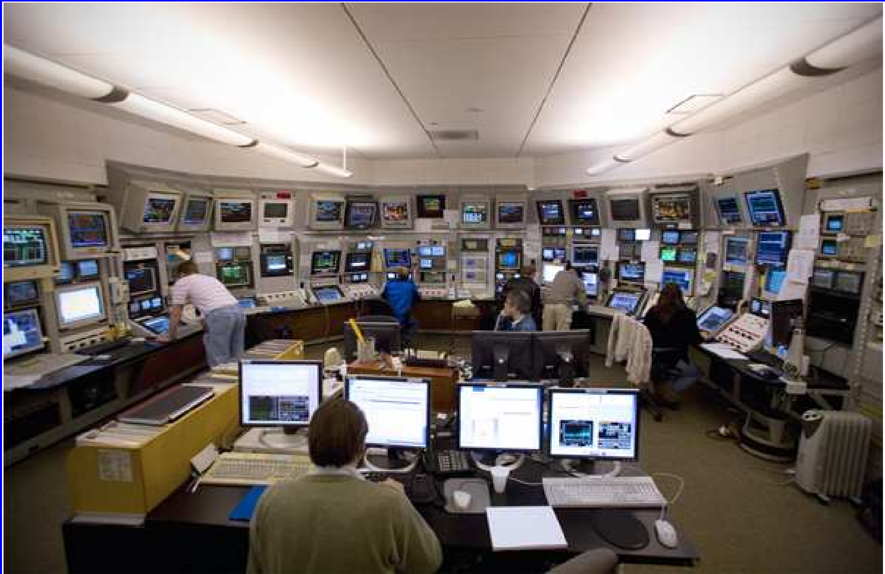
SLAC Main Control Room
