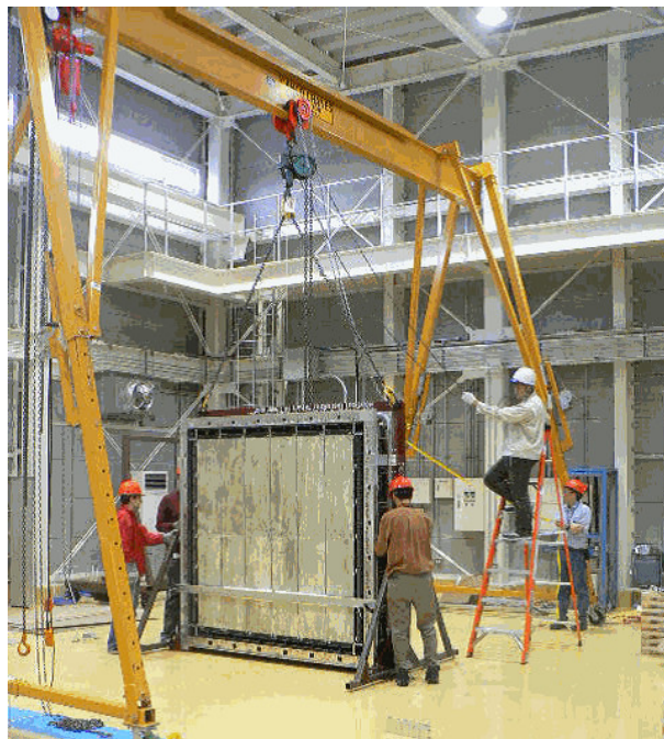
Figure 4.2: Tilting the FGD to the vertical. All assembly works were done by muscle power.
